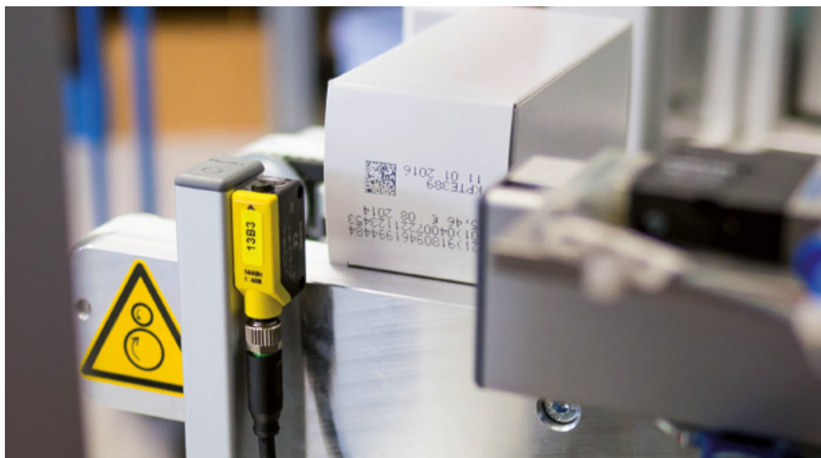
This photoelectric sensor at the reject area of the PALC unit is used to verify the rejection
